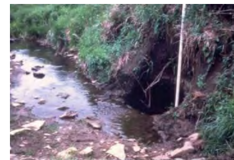
Karst conditions: Water wells in stream sinkhole. Photo Credit: Iowa DNR
